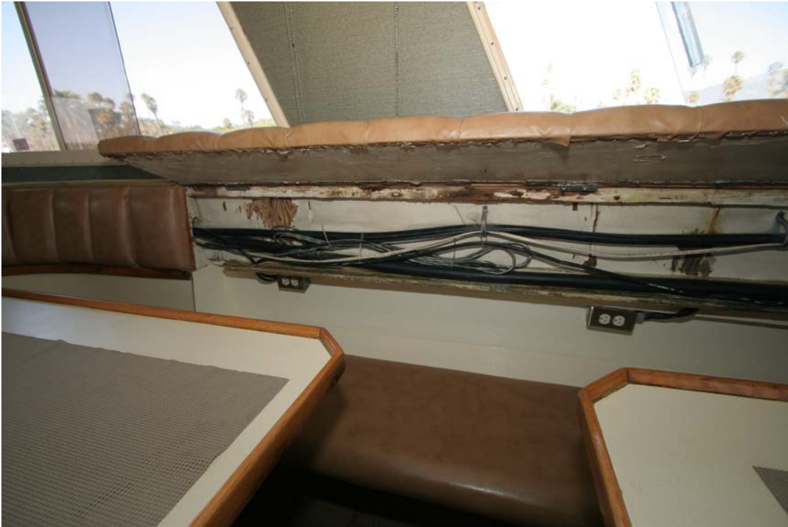
Figure 33. Cable run behind the starboard-side bulkhead seating of the Vision .
