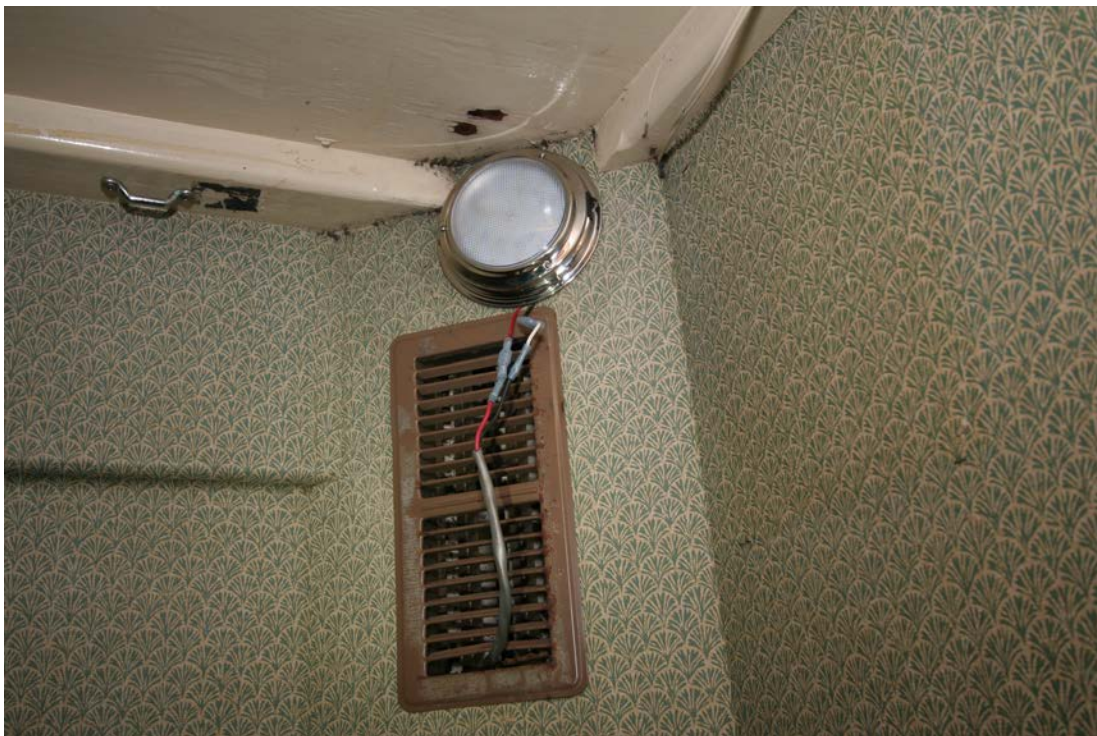
Figure 34. Power cable for lighting routed through ventilation grille in the Vision bunkroom.
